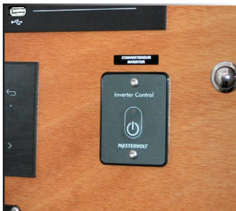
VOLTAGE CONVERTER SWITCH
