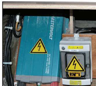
VOLTAGE CONVERTER + VOLTAGE CONVERTER AUTOMATIC BREAKER
