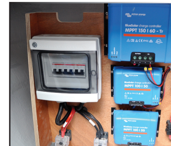
SOLAR PANEL AUTOMATIC BREAKERS
