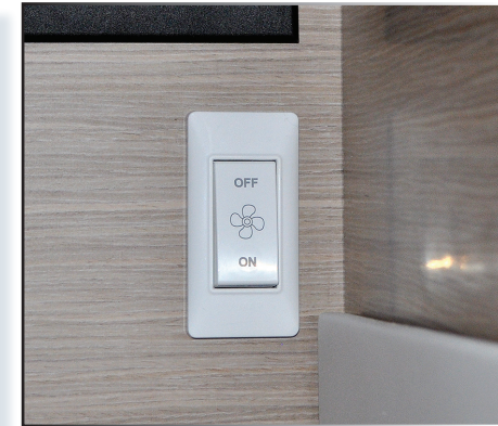
AIR CONDITIONING VENTILATION SWITCH (CABINS)
