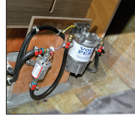
GENERATOR DIESEL FUEL FILTER
