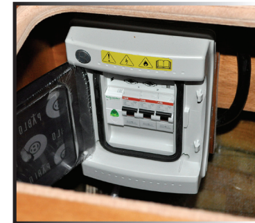
AUTOMATIC BREAKERS FOR AIR CONDITIONING COMPONENTS
