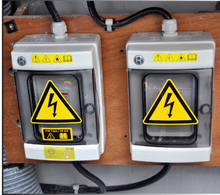
SHORE POWER SOCKETS - AUTOMATIC BREAKERS
