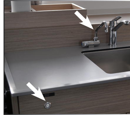
SEAWATER TAP + SEAWATER PUMP SWITCH
