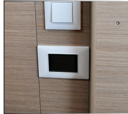
AIR CONDITIONING CONTROL
