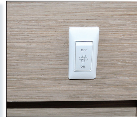
AIR CONDITIONING VENTILATION SWITCH (CABINS)
