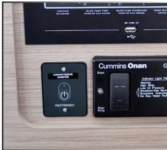
VOLTAGE CONVERTER SWITCH
