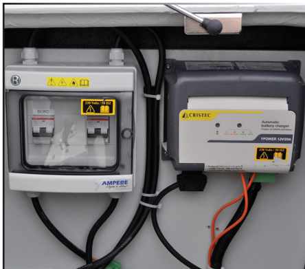
GENERATOR AUTOMATIC BREAKERS + CHARGER
