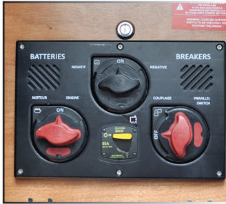
CUT-OUTS FOR BATTERY COUPLINGS, PORT ENGINE AND WATERMAKER
