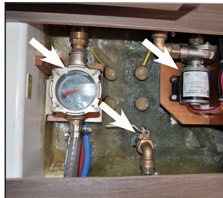
VALVE + WATER FILTER + GENERATOR PUMP
