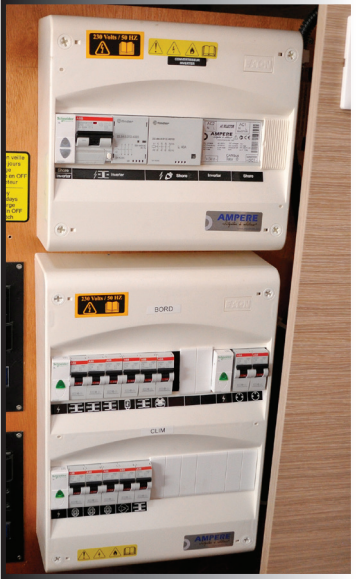
CONSUMING APPLIANCES AUTOMATIC BREAKERS
