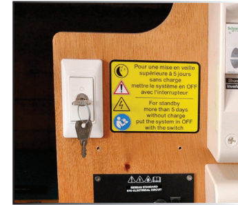
CHANGEOVER SWITCH FOR THE LITHIUM BATTERIES BANK (OPTION)
