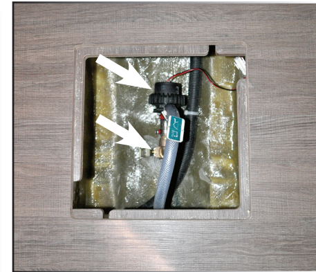
WATER INLET + WATERMAKER BOOSTER PUMP
