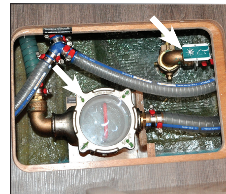
FILTER + SEA WATER VALVE
