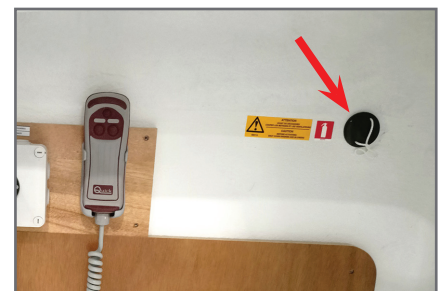
Access to the generator compartment plug
