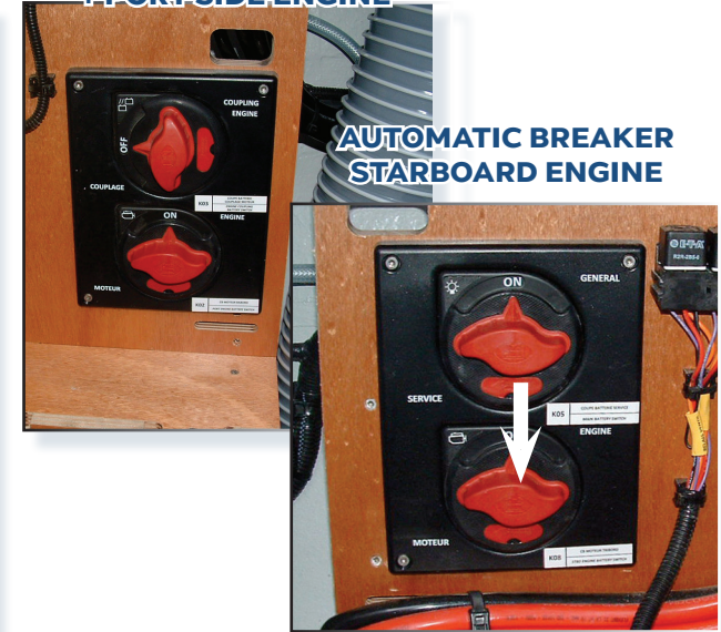
CIRCUIT BREAKER FOR COUPLING + PORT SIDE ENGINE
