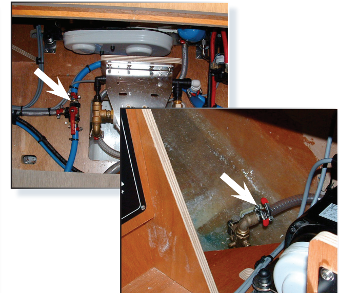
THREE-WAY VALVE + SEA WATER SUPPLY VALVE
