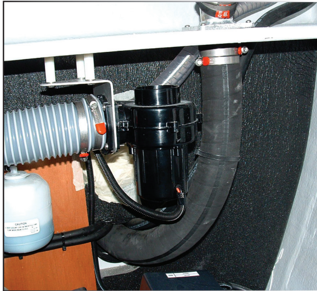
ENGINE COMPARTMENT VENTILATOR
