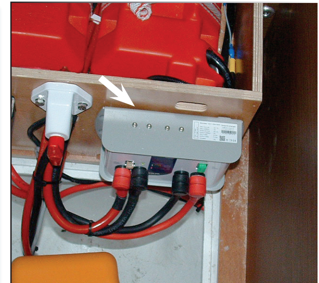
BATTERY CHARGER FOR THE THRUSTER
