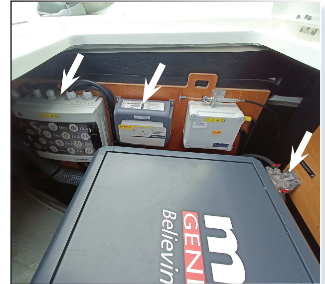
CIRCUIT BREAKERS + CHARGER + FUEL FILTER
