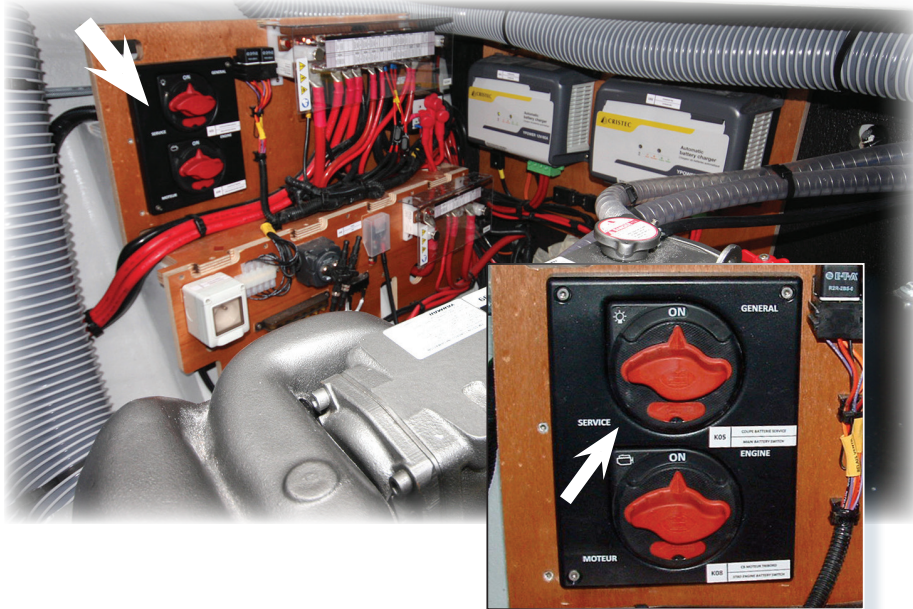
GENERAL CIRCUIT BREAKER STARBOARD ENGINE COMPARTMENT
