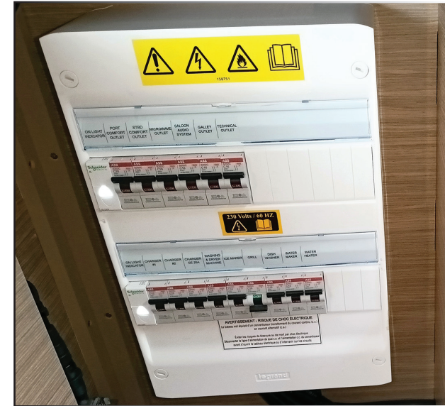
CIRCUIT BREAKERS ELECTRIC CONSUMERS
